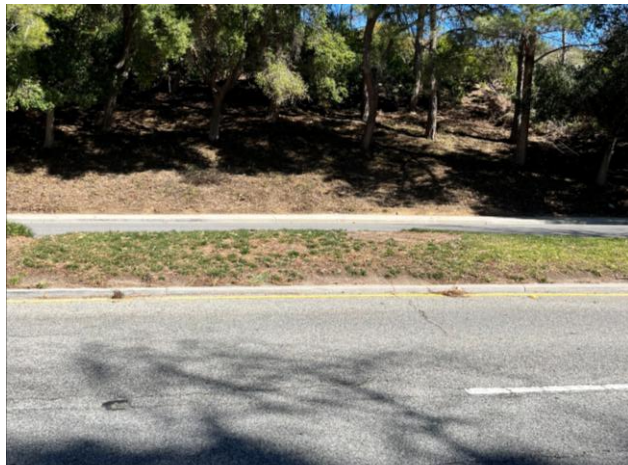
Large slope above Kanan Road. West of Los Arcos Road and East of Golden Eagle Road. Plant material aged out and sparse. Need refresh.
