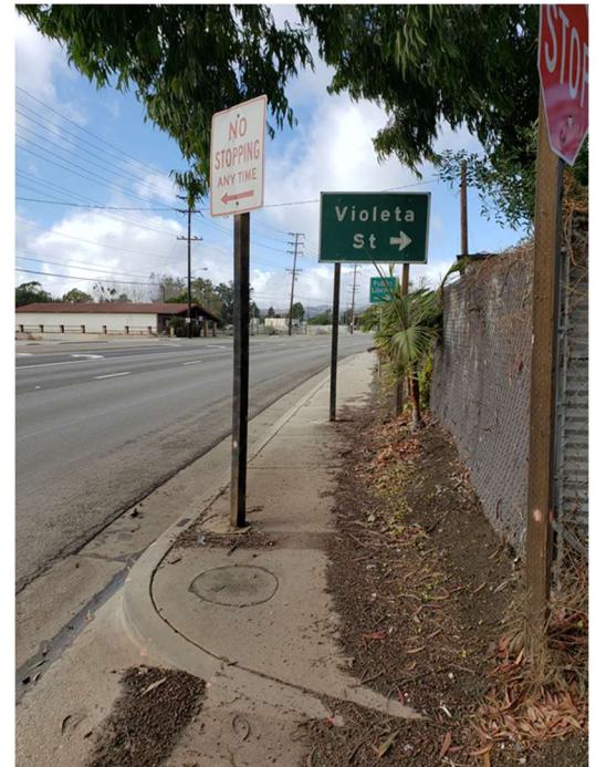
Existing sidewalk conditions on Highway 118 include debris and sign barriers which pose challenges to pedestrians and people with strollers or in a mobility device. Photo taken on Highway 118 near Violeta Street.
