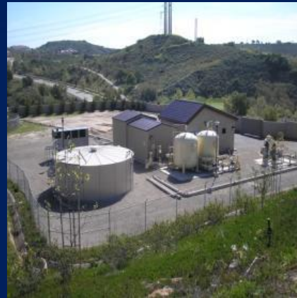
WWD No. 1 Well No. 20 with wellhead treatment
