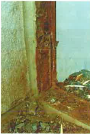
A severely deteriorated frame, such as this, can be replaced in kind. Photo: Henry Chambers, AIA.
