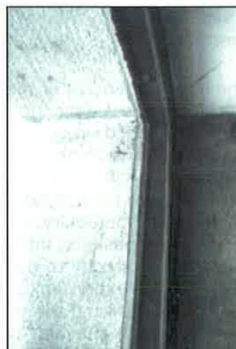
This is a successful replacement in kind of the deteriorated frame shown above. Photo: Henry Chambers, AIA.
