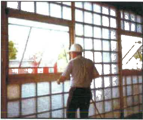
Maintaining historic steel windows for continued use is always recommended. Photo: NPS files.
