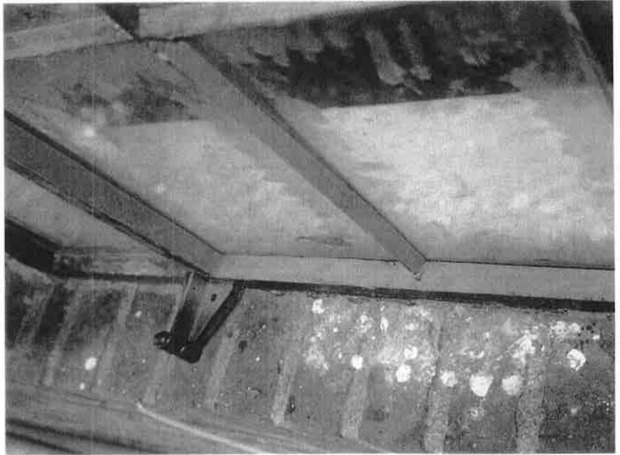
Figure 9. An oil-based putty was used to reglaze the historic casement windows. Painting was undertaken two weeks after reglazing.
