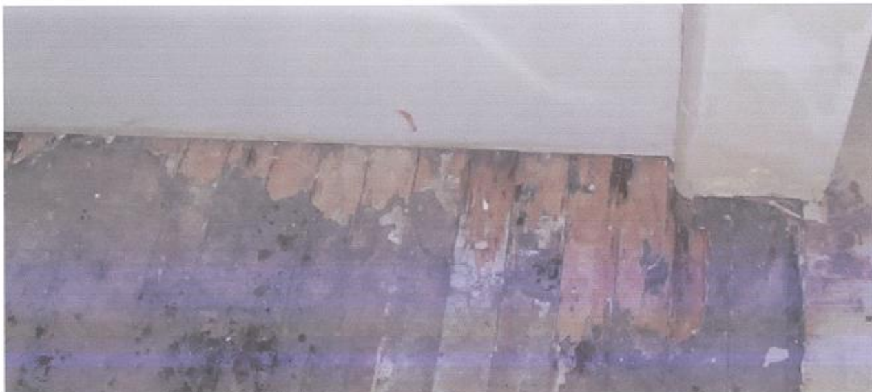
Termite damage under the vinyl flooring in the bathroom.
