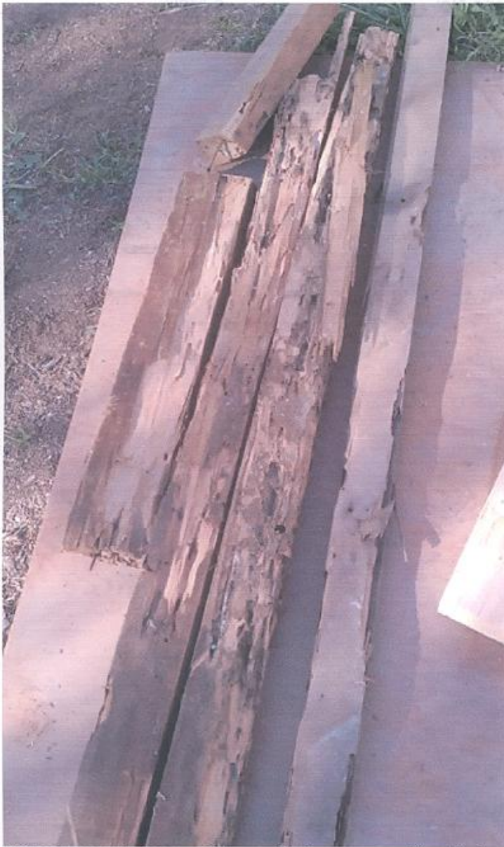
This is an example of some of the wood that was removed from the house and replaced.
