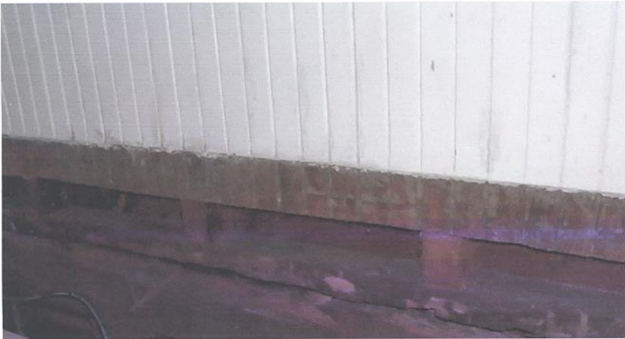
This photo shows the condition of the sub floor and wall in the laundry room as we were removing the boards that were unusable.
