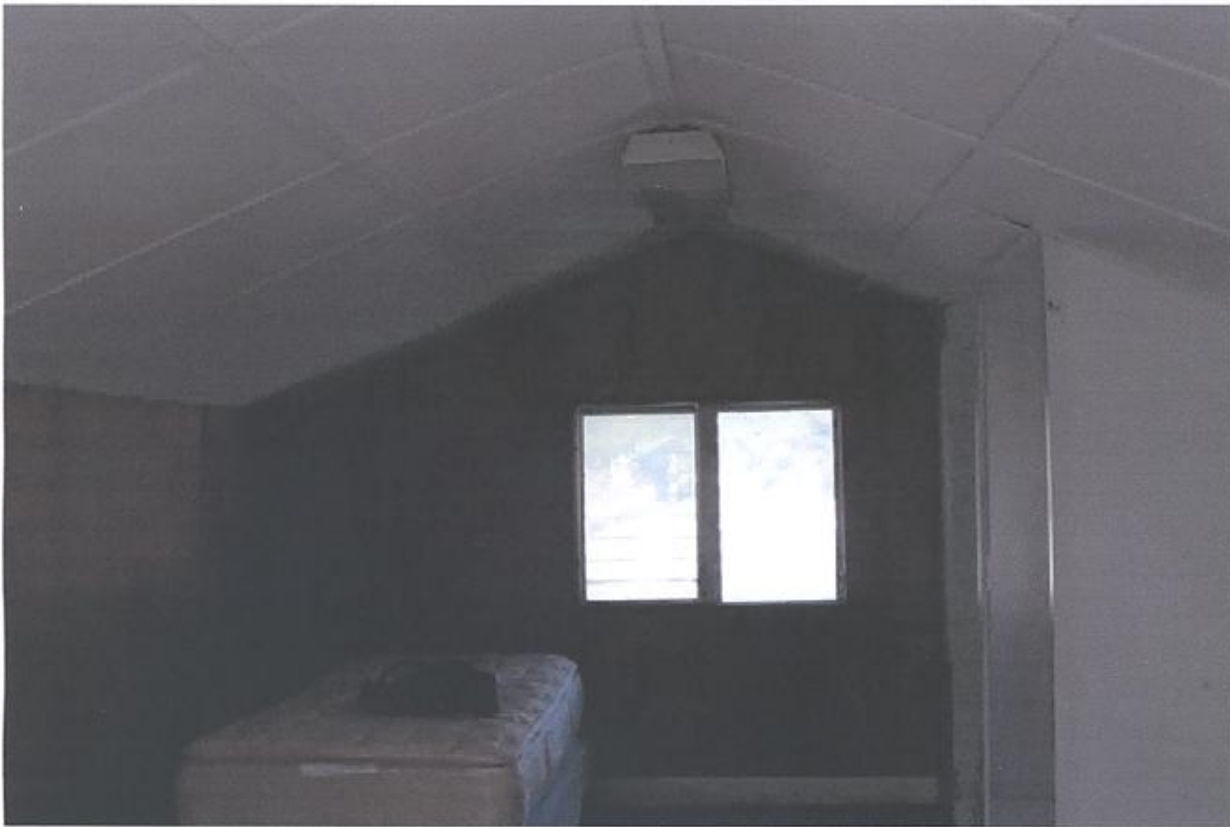
Upstairs, we removed the paneling, the drywall behind it, the beaver board on the ceiling and the carpet. We would like to replace these aluminum windows with wood or wood clad and turn the closet you see here into part of a second bathroom for the house.
