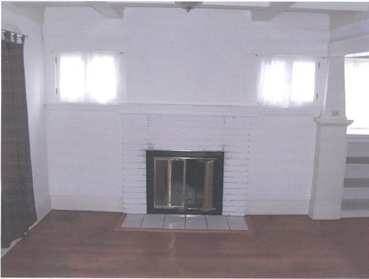
We removed the fireplace doors and the hearth tile on the floor and the popcorn on the ceiling.
