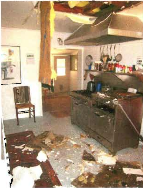
Photo shows collapsed ceiling in 2009 winter rains
