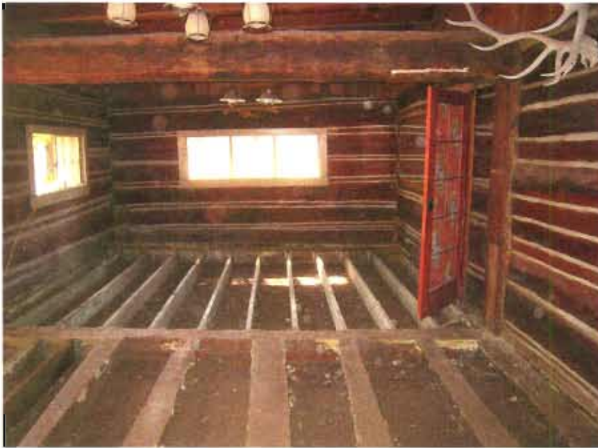
Dining room area – floor joists logs were replaced a 1990's repair
