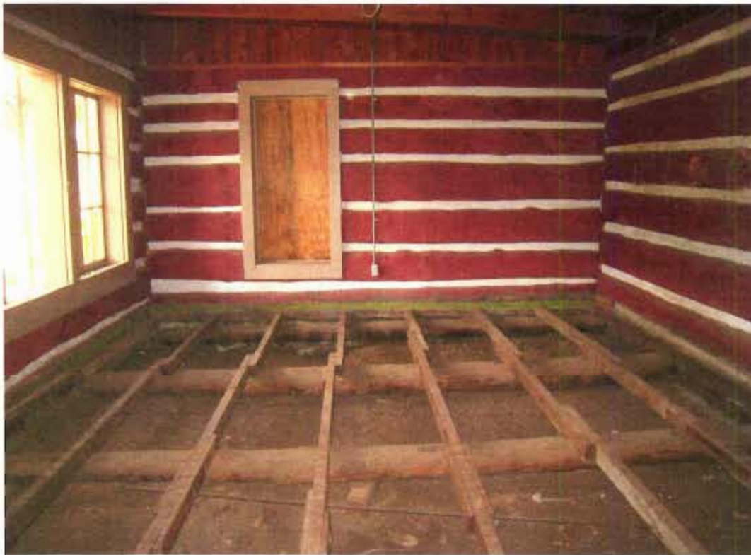
Bedroom #1 – log floor joist modified with added lumber at some time in the past
