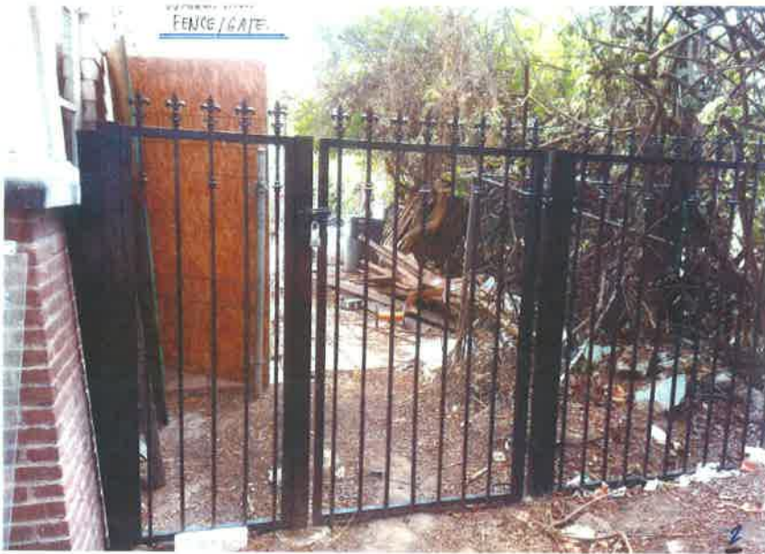
Photo No. 4 taken from front yard in 2016 of wrought iron fence and gate at west elevation
