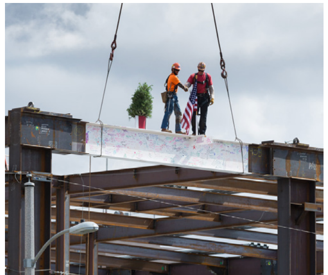
The 'Topping Off' ceremony, a tradition in the construction industry, marks the last beam in place milestone.
