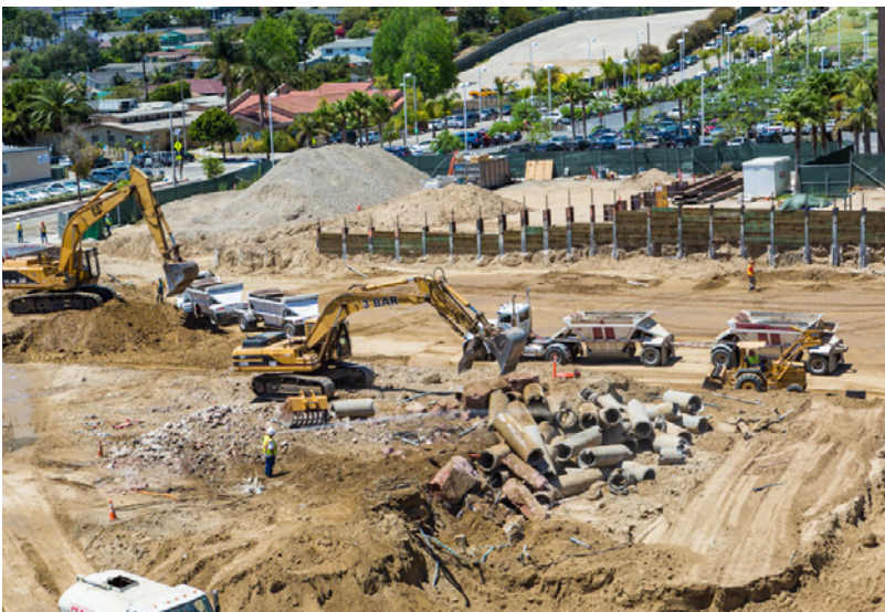
The VCMC Hospital Replacement Wing Project is ahead of schedule, with some units opening as early as fall 2016.
